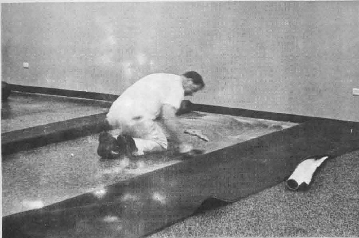
Oblivious to all but his work, a carpet layer installs new carpeting on the third level of the library. However, library officials don't expect the carpeting to be much help in their daily battle to control the noise level.
